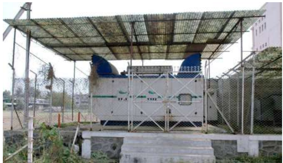
Any other facilities (Electrical Generator)
